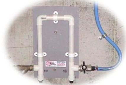
Typical Corrosion coupon rig
